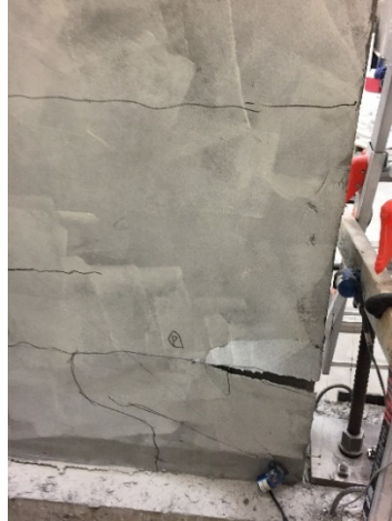
(b) Toe crushing.
