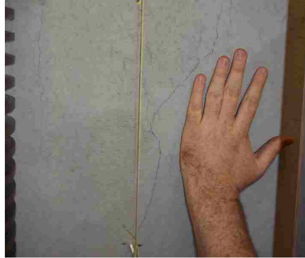
(b) Close up view of crack on wallette face.
