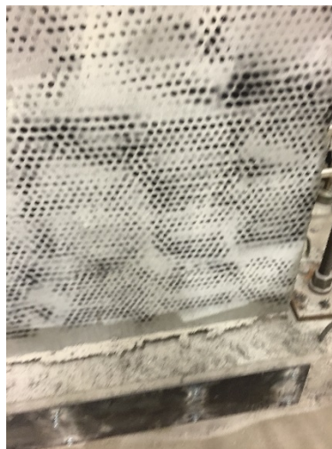
(b) Wall uplift.
