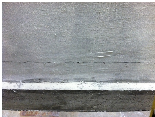
(b) horizontal crack.
