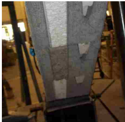
(b) Cracks in web after testing.
