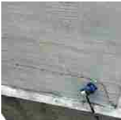
(a) Toe crushing and horizontal crack.
