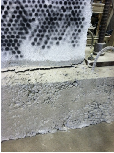
(a) Uplift of wall.
