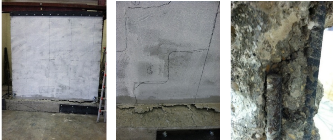
(a) Uplift of wall. (b) Typical diagonal cracks. (c) Pullout of dowel from grout.
