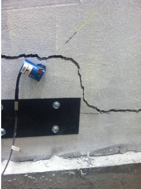
(a) Failure around steel plate.
