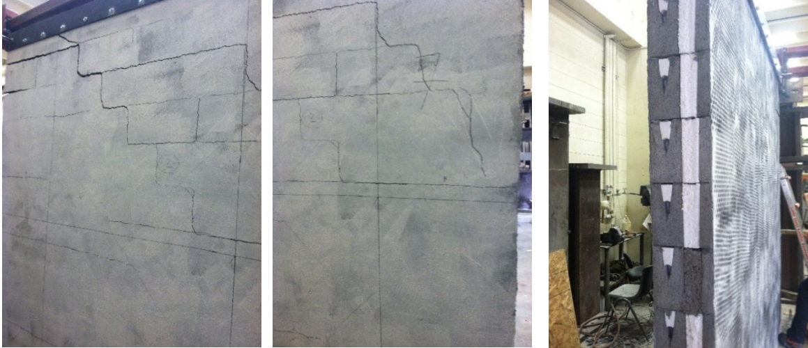
(a) Opening in top course. (b) Typical diagonal cracks. (c) Lack of cracks in webs.
