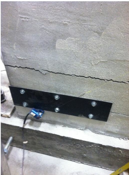
(a) Horizontal crack above steel plate.
