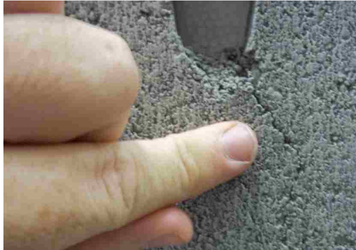
Figure 4-7 Cracking in web prior to testing.
